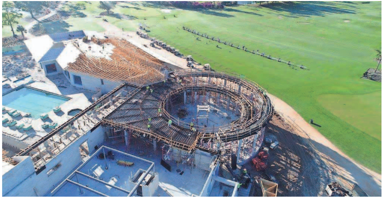
A drone's perspective shows the renovation project currently underway at Quail Creek Country Club. BROOKE SELVIDIO/DON GARRETT CONSTRUCTION
